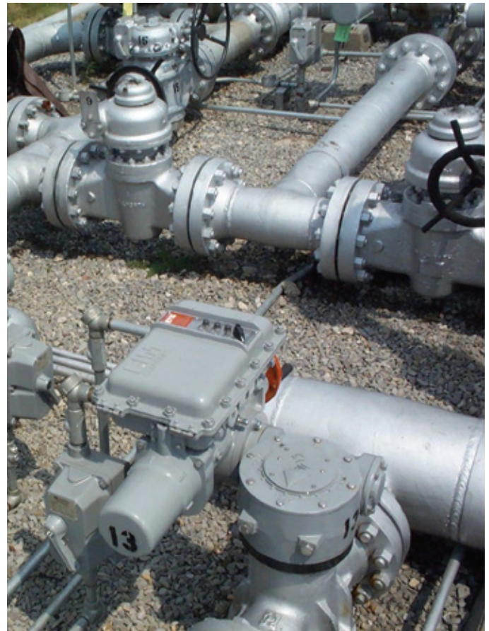
Actuators in gas compressor stations must operate under constant vibration.
