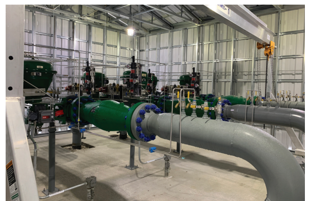
Fig. 1. Natural gas pipeline pressure reduction applications often employ two valves in a worker/monitor configuration, as shown in the left figure. The downstream gas pressure will not significantly change if one of the valves fails, as each is designed to provide the full amount of required pressure reduction. (Credit: All Figures courtesy of Emerson)
