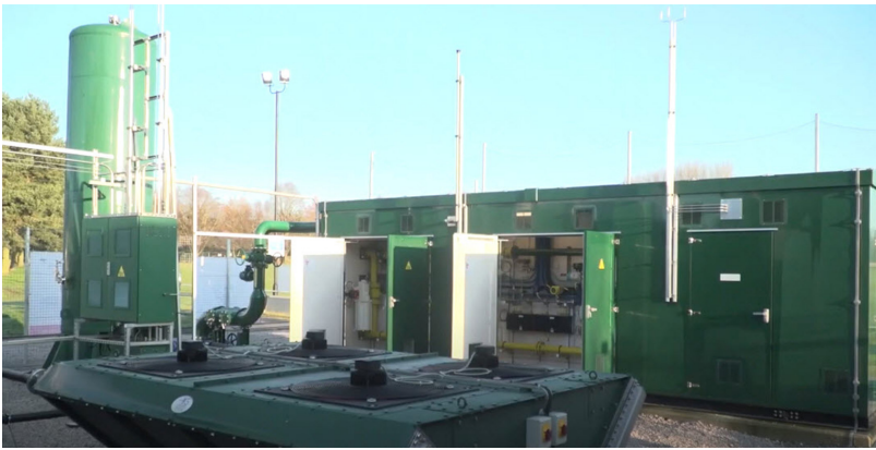
Figure 2: Green hydrogen is stored in the buffer tank before it gets mixed with natural gas and injected into the natural gas network.
