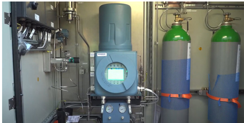
Figure 1: The HyDeploy project uses Emerson's Rosemount 700XA Gas Chromatograph to provide independent validation of the full hydrogen and natural gas blend rate.
