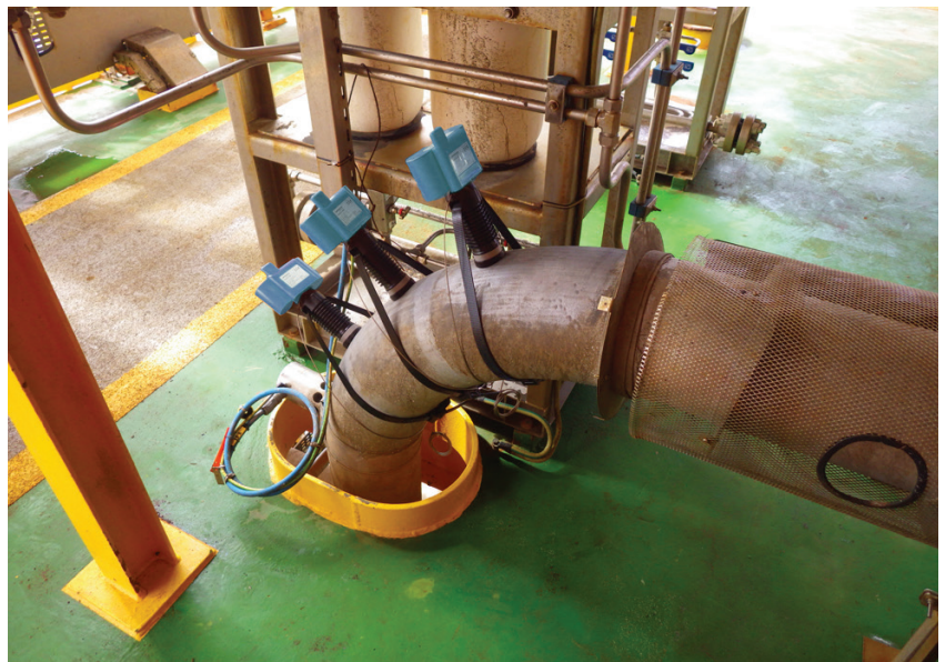
FIG. 3. Wireless non-intrusive thickness sensors installed in an offshore environment.
