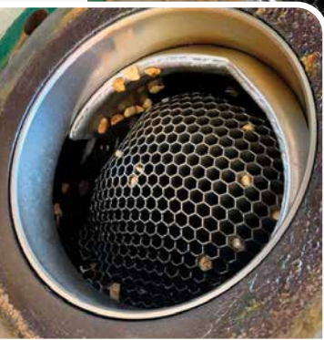
Figure 6: The anti-cavitation trim was replaced with a higher hardness R31233 alloy and returned to service for another year. The inspection team found a few small rocks stuck in the trim, but no damage to downstream piping, no damage to the valve body and reduced erosion damage of the Hex trim. Image courtesy Emerson
