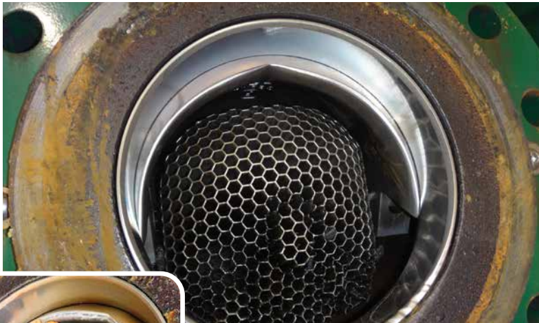
Figure 5: After a year in service there was no sign of downstream piping damage and damage was limited to relatively minor erosion on the face of the trim. The valve body suffered no damage at all. Image courtesy Emerson
