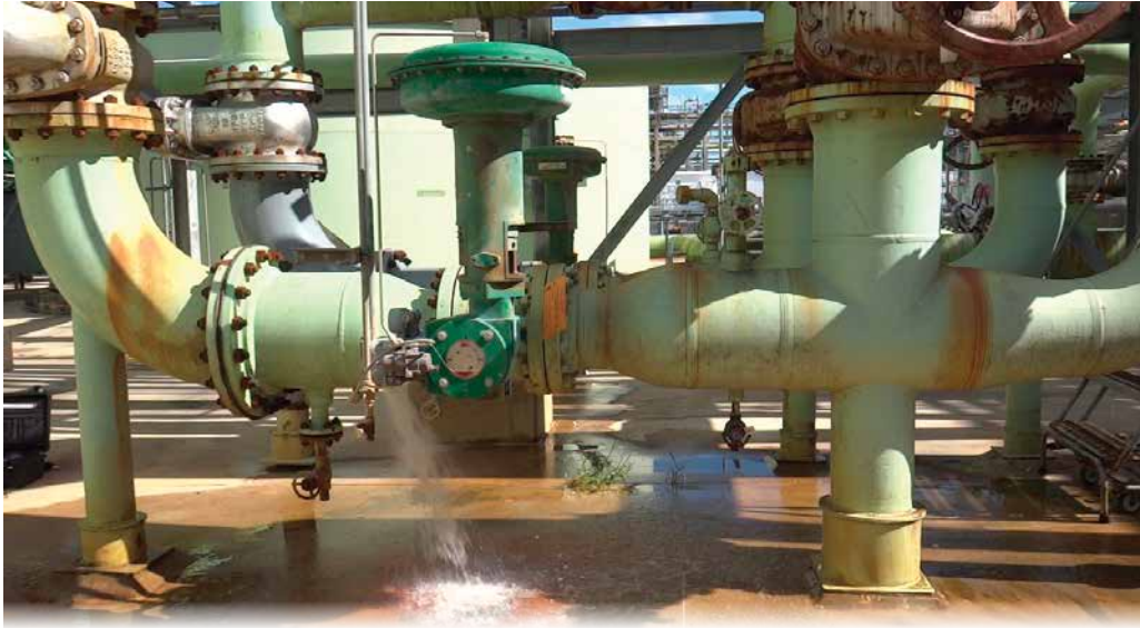
Figure 2: Downstream piping fails due to extreme cavitation and the erosive effects of river silt striking the pipe wall. Note the river water spraying out of the pipe at the bottom left of the photo. Image courtesy Emerson
