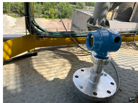
Image 1. Rosemount 5408 Non-Contacting Radar Level Transmitter installed on top of the sand tank
