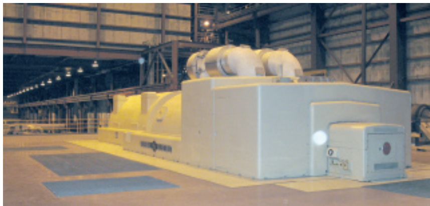
2. Nominal 100-MW steam turbine guards one end of the building and looks down on the gas-turbine "alley"
